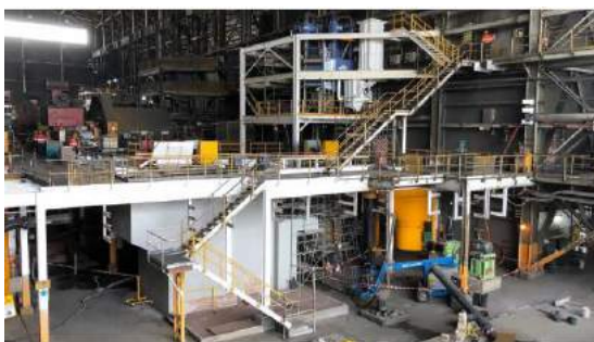
The copper concentrator plant in 2020
