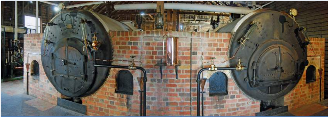
Figure 1: The boiler house at Sovereign Hill with both century-old boilers banked for the night.
