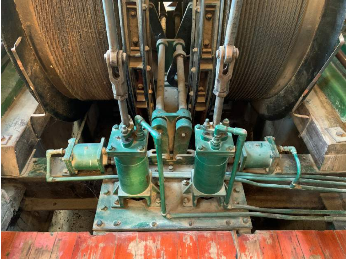
Figure 3: The air actuation system. The vertical cylinders control the winder brakes, the horizontal cylinders control the drum clutches.
