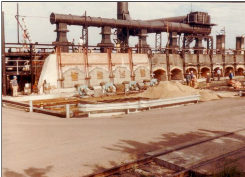
Figure 4: New ovens and flue system. Taken on 27 August 1984, the photograph shows the beginning of the common flue system and the bottom half of the southern stack
