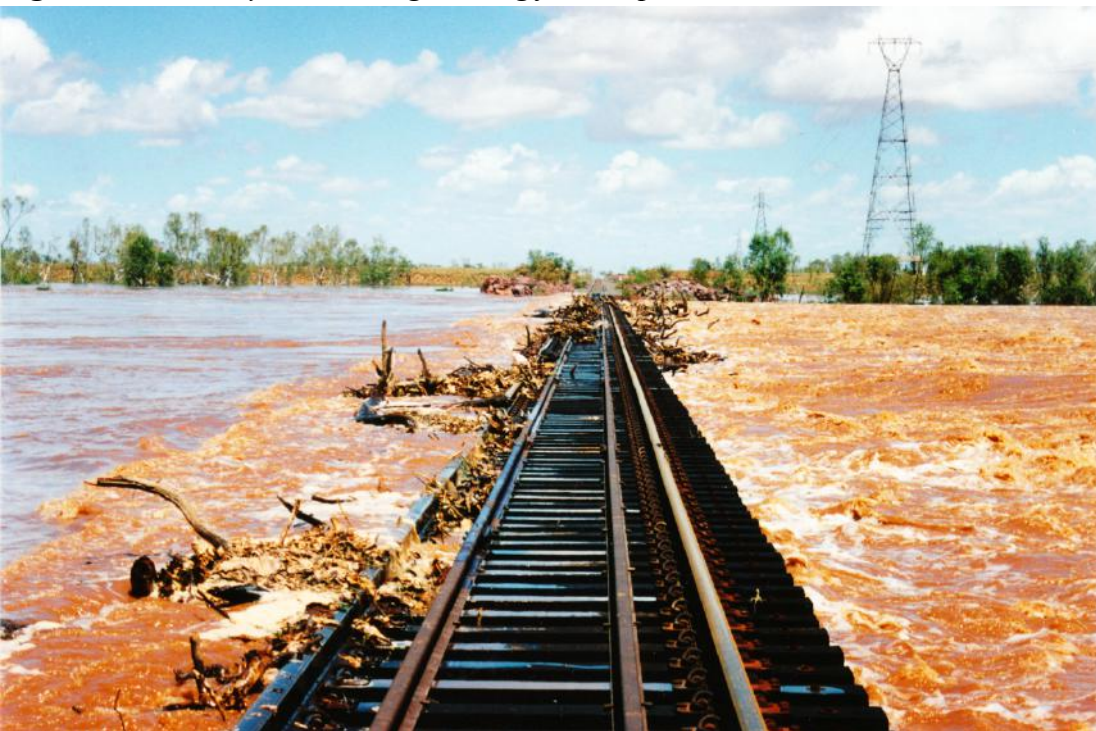
Figure 1A: De Grey River Bridge during flood, April 1996.
