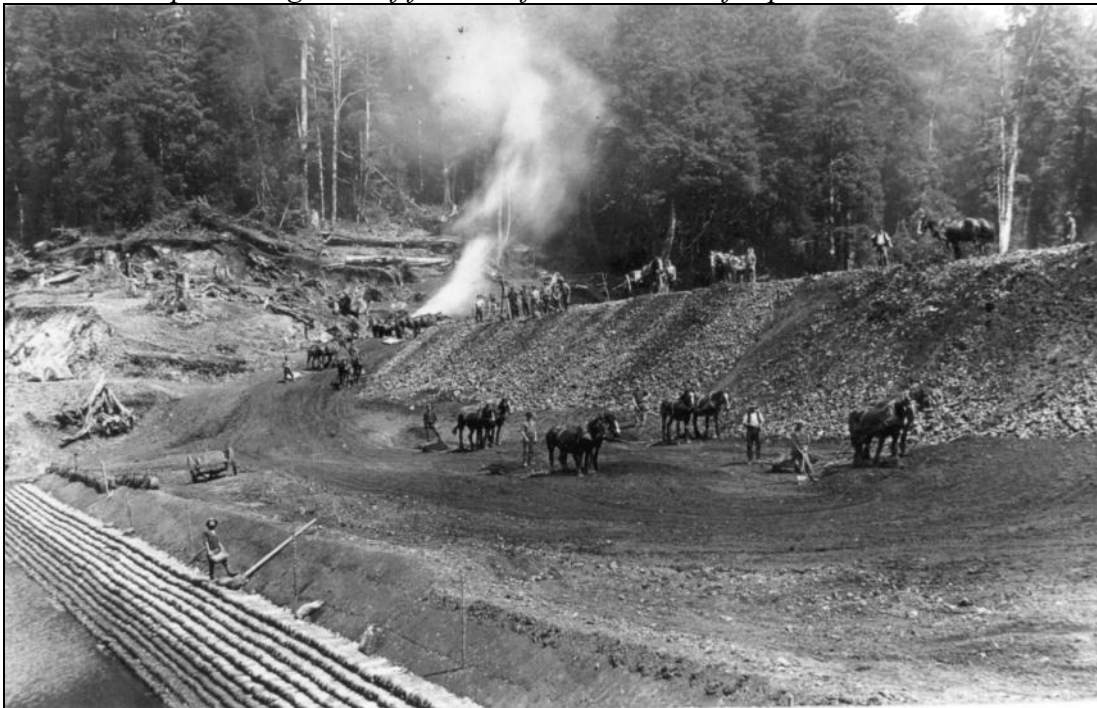
Figure 3: No. 2 Dam during construction – sandbag lining on the upstream face of the embankment protecting zone of fine rockfill, coarse rockfill placed on downstream side.
