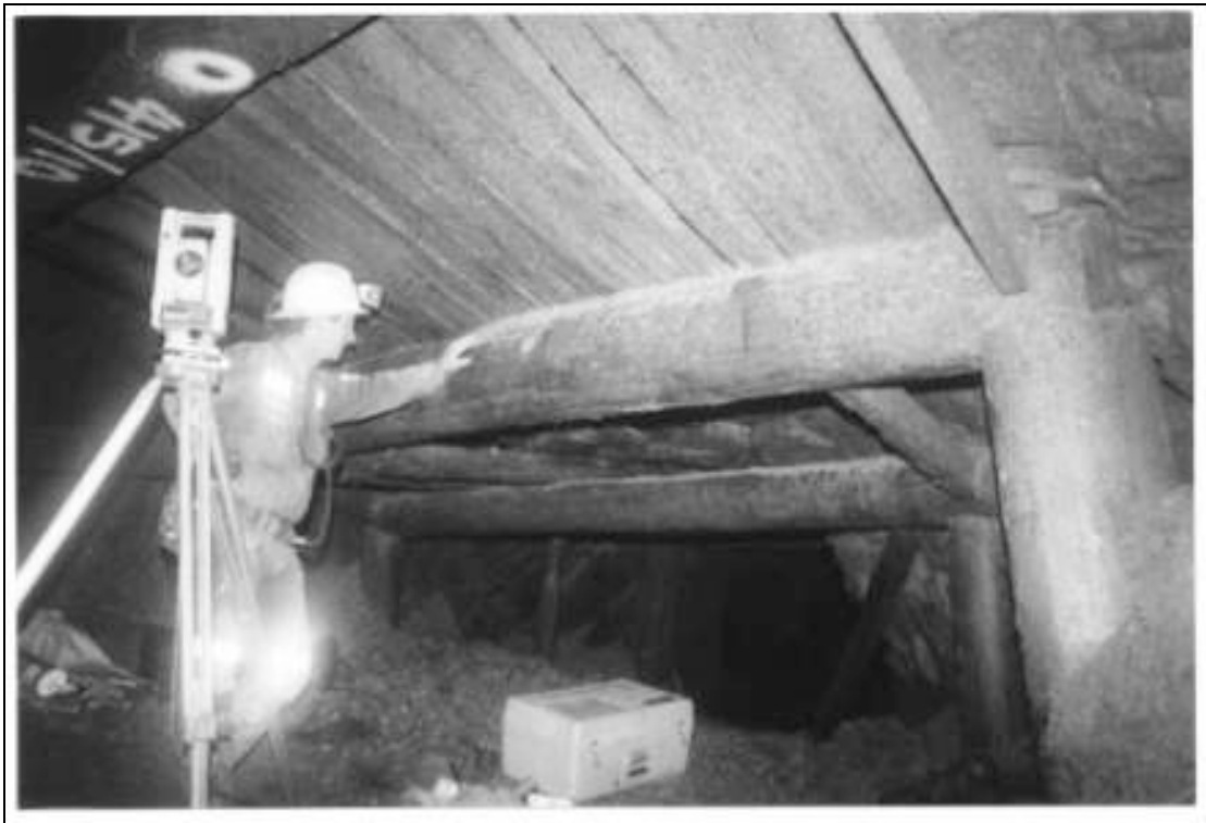
Figure 3: Timber lining and backs support in the plat area in front of the winding compartment, as it appeared on 4 July 1998.
