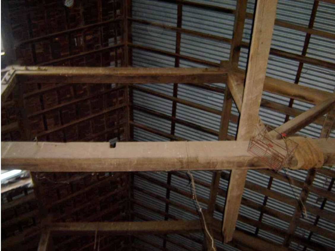
Figure 9: Roofing timbers exhibiting clear loppings-off where supports had extended upwards for the venting clerestory.
