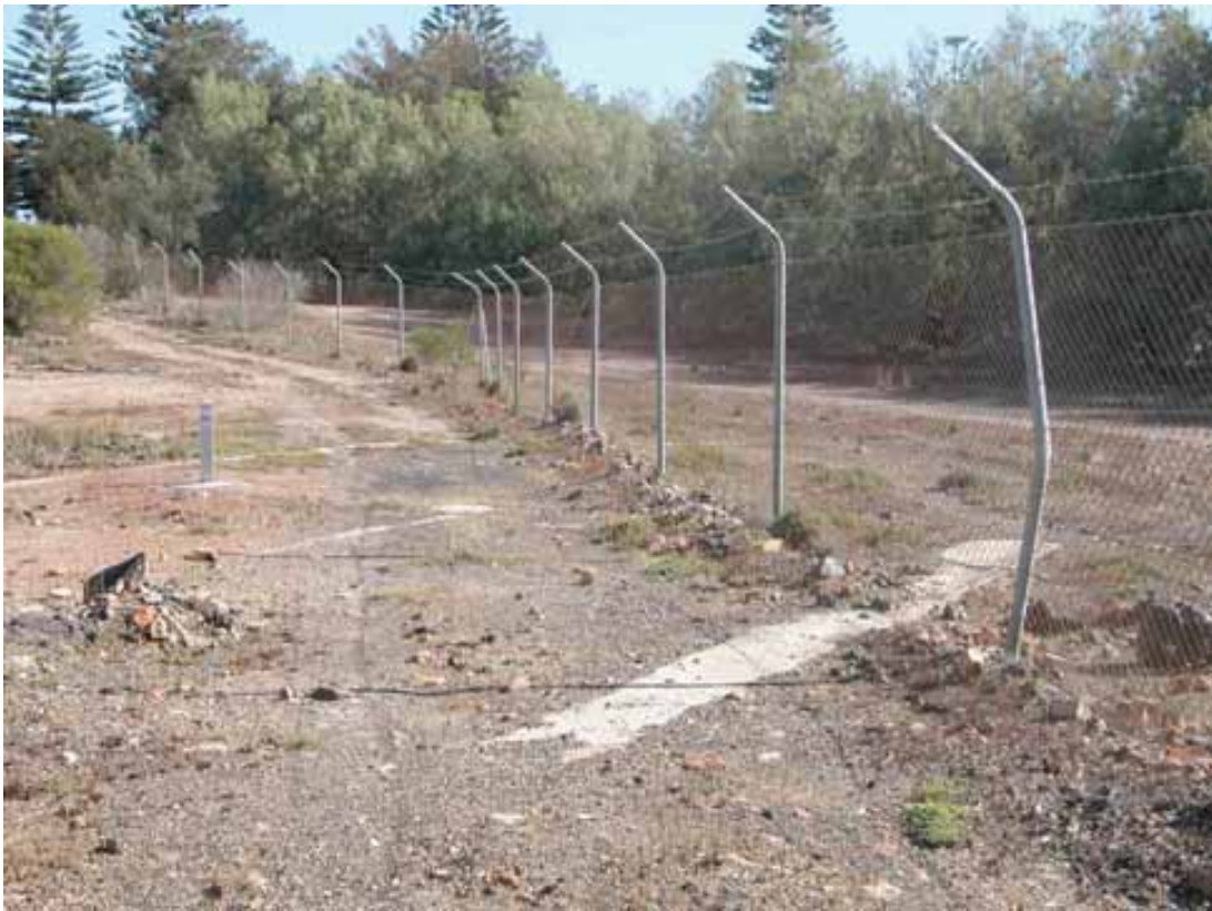
Fig 31 The foundations of the smelters store building extend beyond the project area boundary
