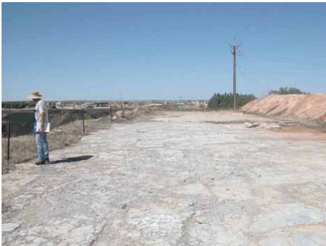
Fig 34 The paved area on the upper level near the north end of the retaining wall is the charge floor where the blast furnaces standing on the lower level (at left) were fed (see Fig 13, p. 21)
