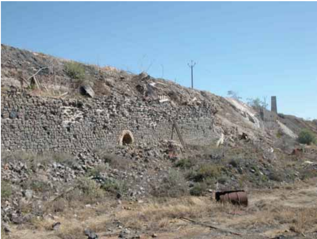
Fig 29 The retaining wall is a dominant element of the site, over six metres high in places, some of its length formed of two walls with internal flues from the furnaces between them
