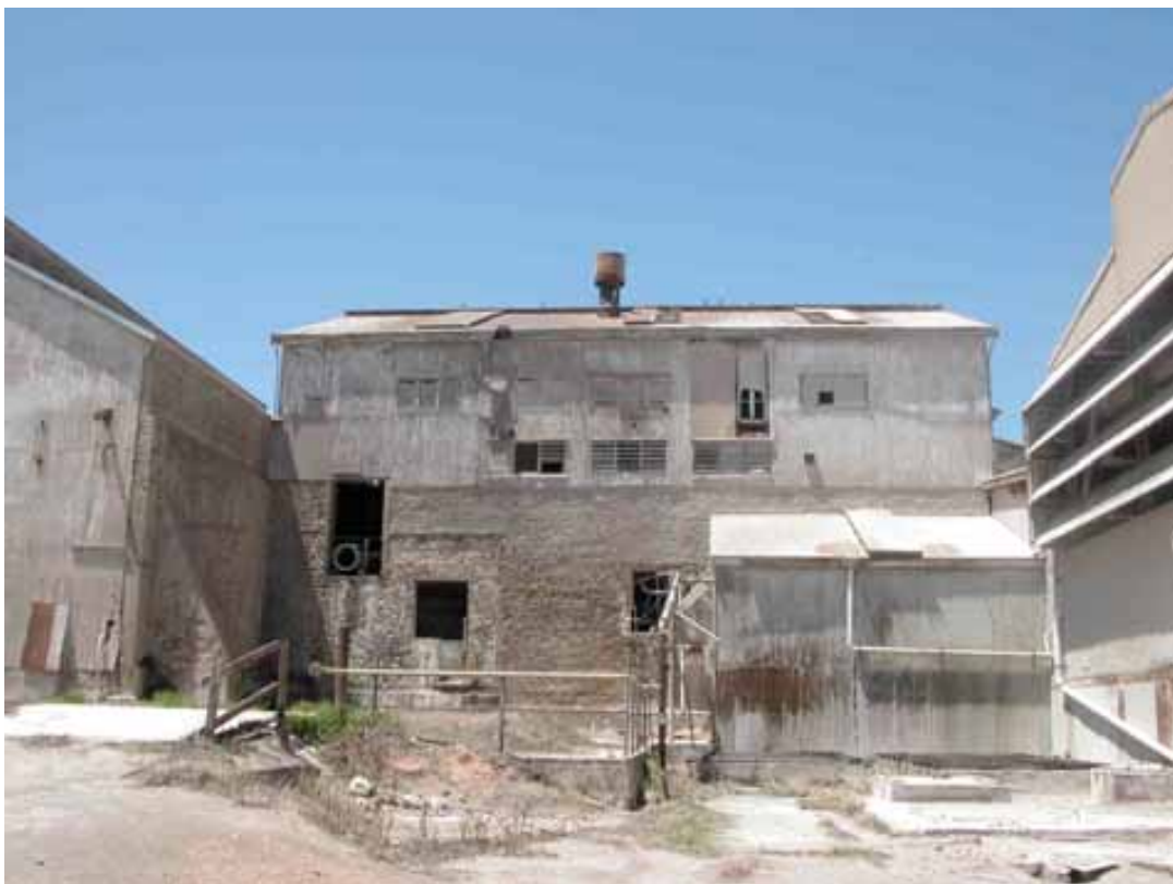
Fig 46 Some stone masonry elements of the original 1900 fertiliser factory still stand, much altered and in poor condition, view from west
