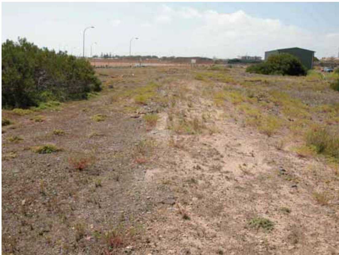
Fig 42 One of the 200m-long coal gantry track foundations, looking north (see Fig. 17, p. 23)
